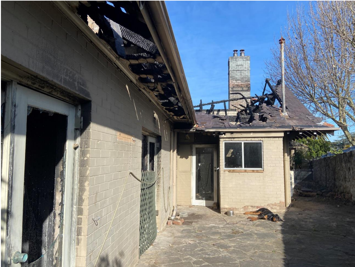
Figure 4 – View of the front house looking west showing burnt-out roof, eaves and loss of slates.
