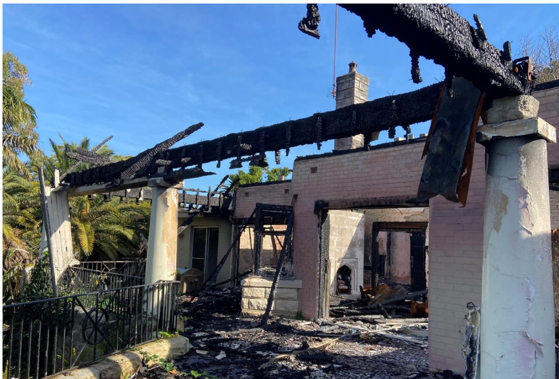
Figure 5 – View of opening to terrace into the house. Floors, joists and bearers have been destroyed, no roof or ceiling, and architraves and door jambs are missing.
