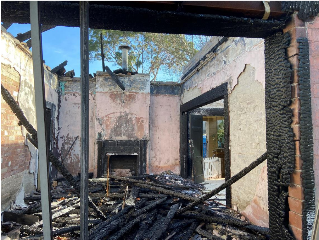
Figure 6 – View east across the south-eastern room. There is no roof, ceiling or floor and architraves and door jambs have been burnt. The fireplace surround is badly charred.
