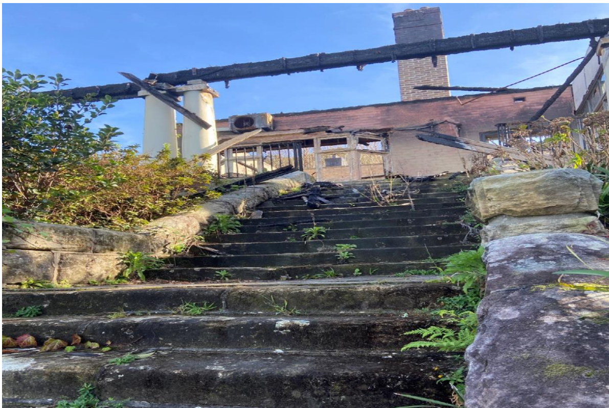
Figure 9 – View from the rear garden of the sandstone stairs and flanking walls looking north dating from the original construction phase.
