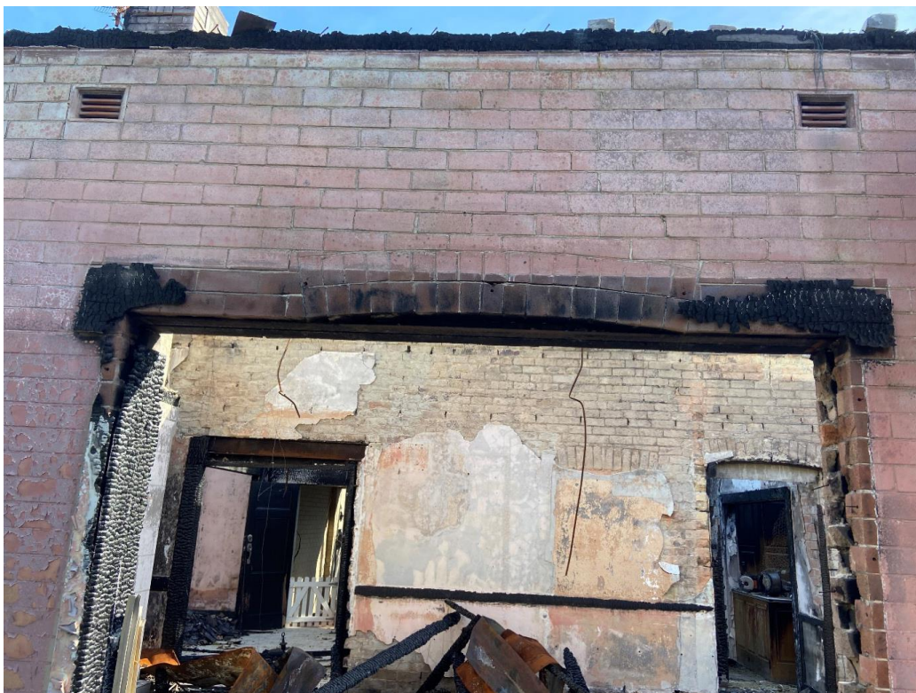
Figure 7 – External opening showing the original arch and steel beam inserted to widen the doors. Cracked and missing wall plaster can be seen on the rear wall.
